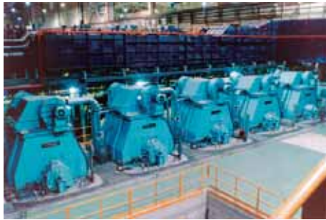
Main electric motors for metal rolling mills
